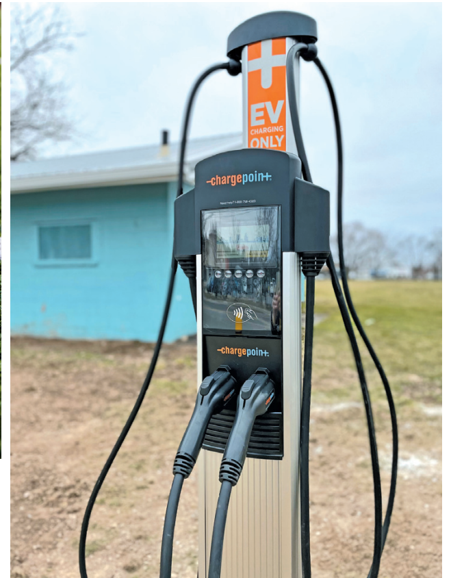
An electric car-charging station was installed this week at Academy Park, just adjacent to the Niagara River Region Chamber of Commerce office and the comfort station.
